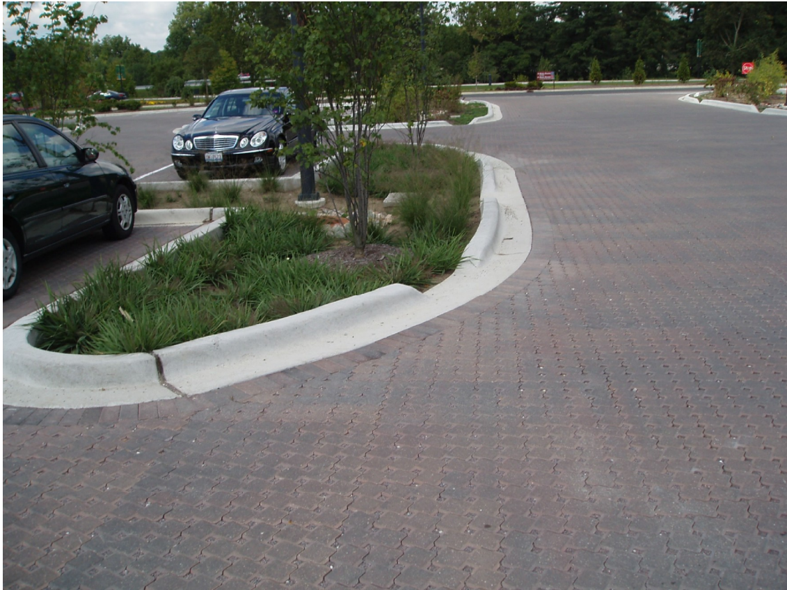
Exhibit 6. Permeable Pavement (Photo from website www.bioretention.com )
